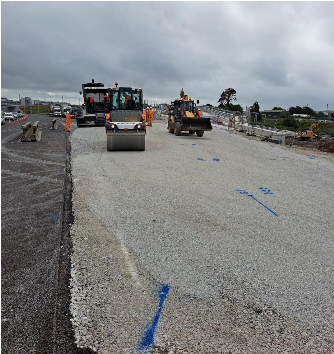
Pavement works ongoing for the Link M tie in at the N25 Westbound Diverge to the Interchange Roundabout.
