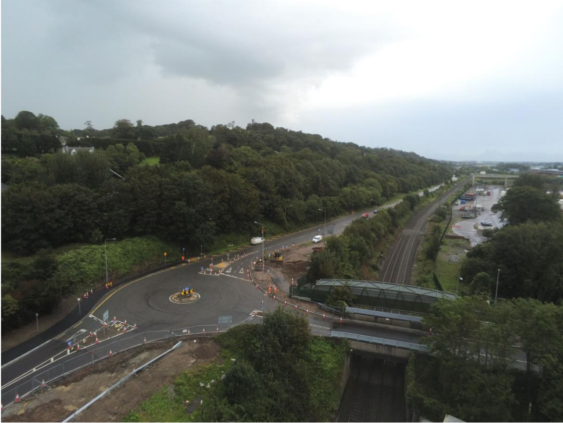
Aerial view of the emerging completed layout at the Bury's Bridge junction area
