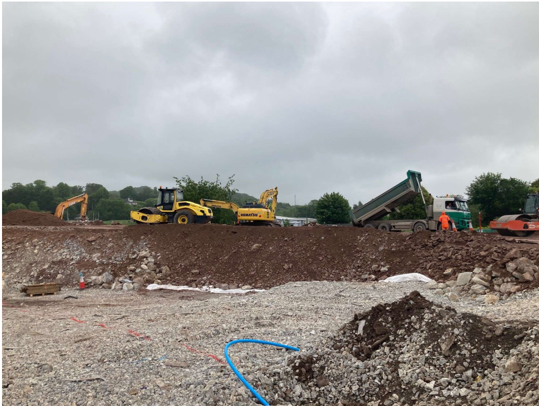
Placing of general fill material to form the road embankments North of the N25 at Link E.
