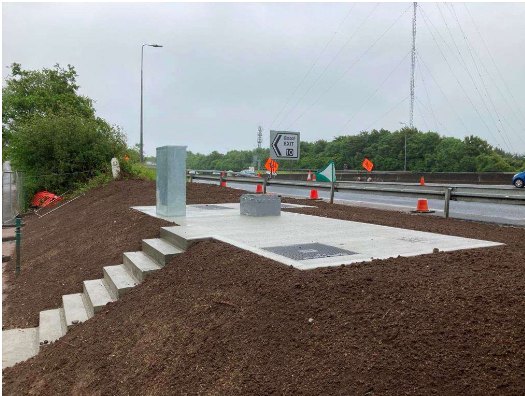
Finishing works completed at an ITS site on the N40 EB diverge for Mahon Point.
