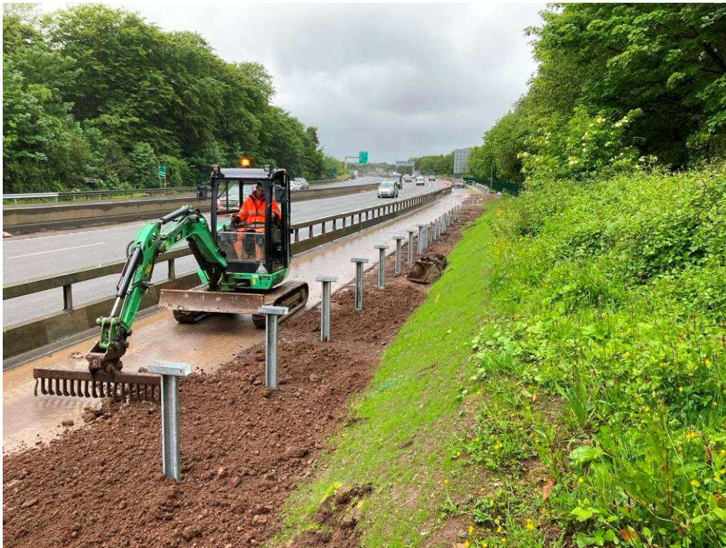
Finishing works being completed around safety barrier posts on the N40 eastbound.
