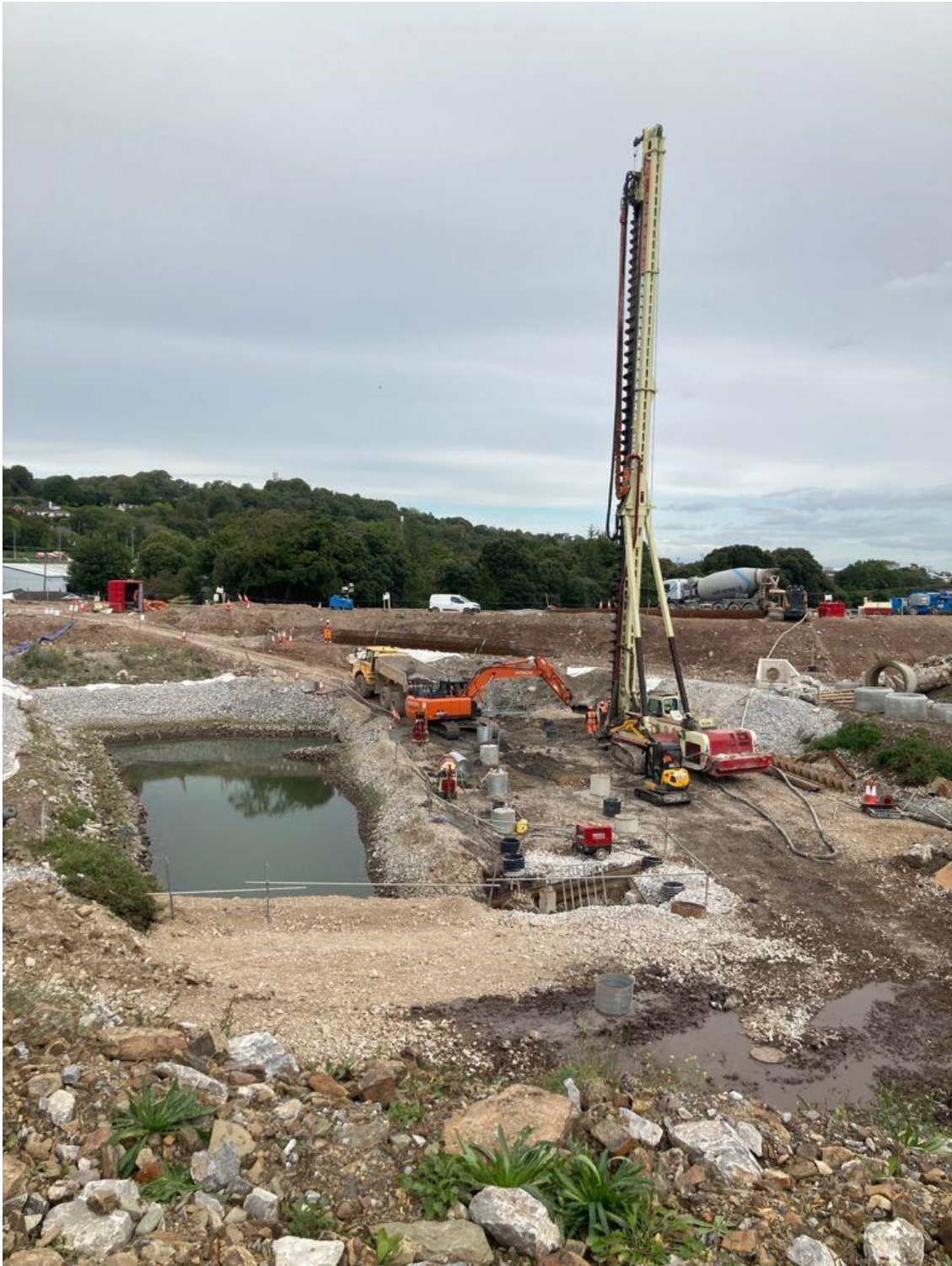
Installation of support piles for Culvert 02 just north of the N25 near the Dunkettle Interchange Roundabout.
