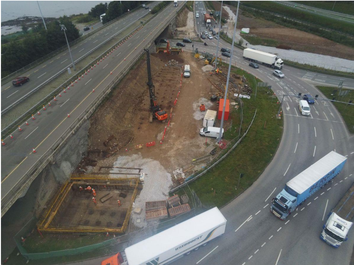
Ongoing ground improvement works at the Interchange centre island area with a concrete pour getting underway.
