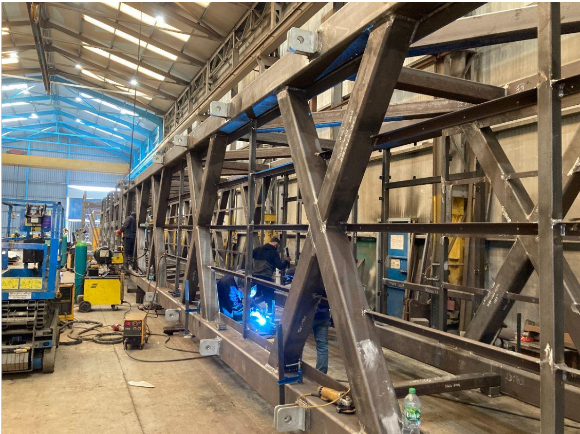
Final stages of fabrication of the 35m span, 56 tonne steel gantry being undertaken
