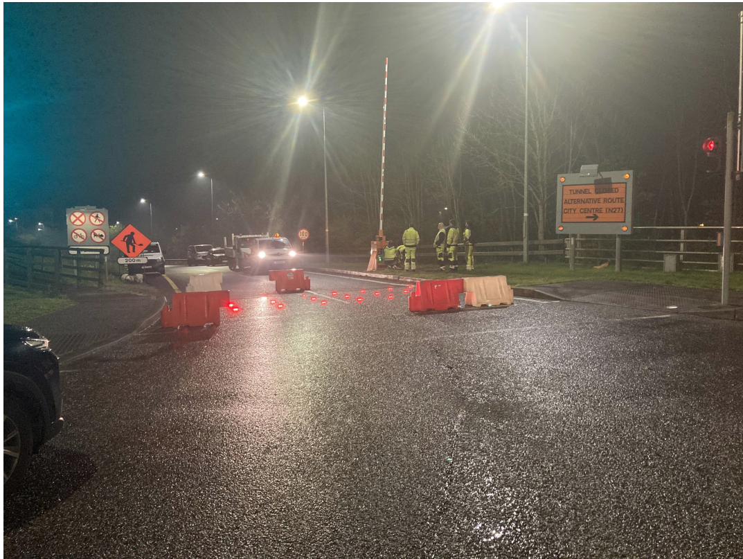
Testing of new barrier and road studs system at the N40 eastbound on-slip from Mahon.
