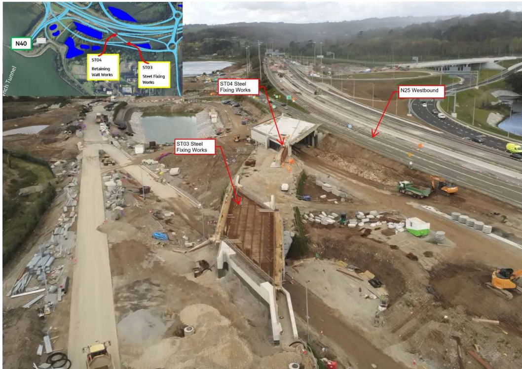
ST03 steel fixing works nearing completion with ST04 Retaining Wall works ongoing also.
