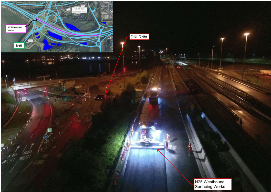
Surfacing works being undertaken on the N25 Westbound in the vicinity of the Interchange Roundabout.
