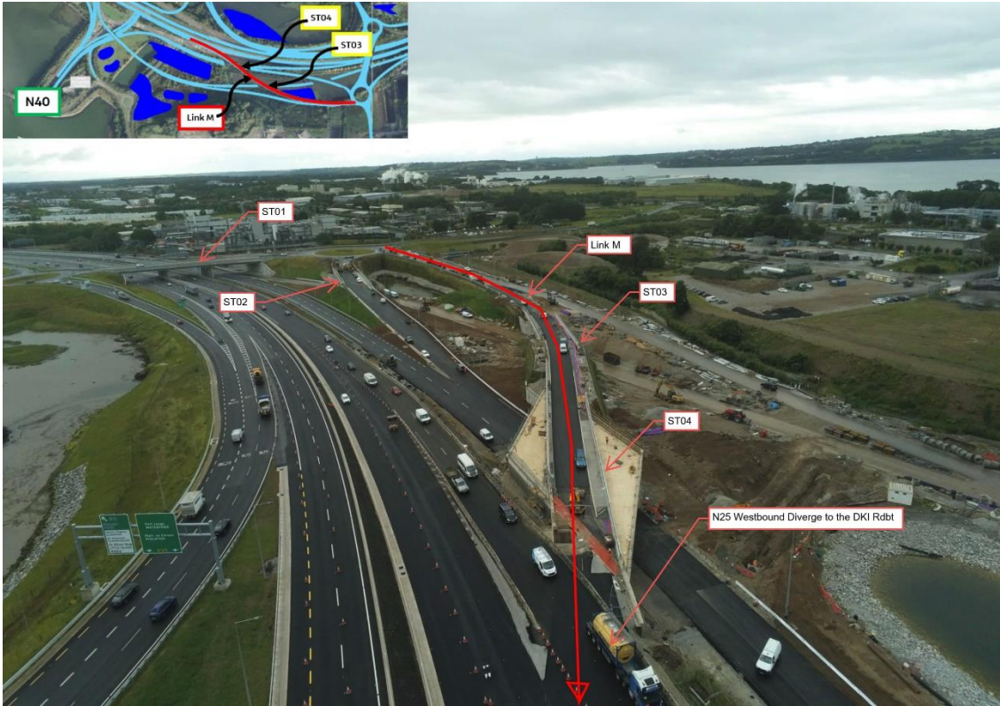
Link M temporary tie in works completed across the N25 Westbound Diverge to the Interchange Roundabout.
