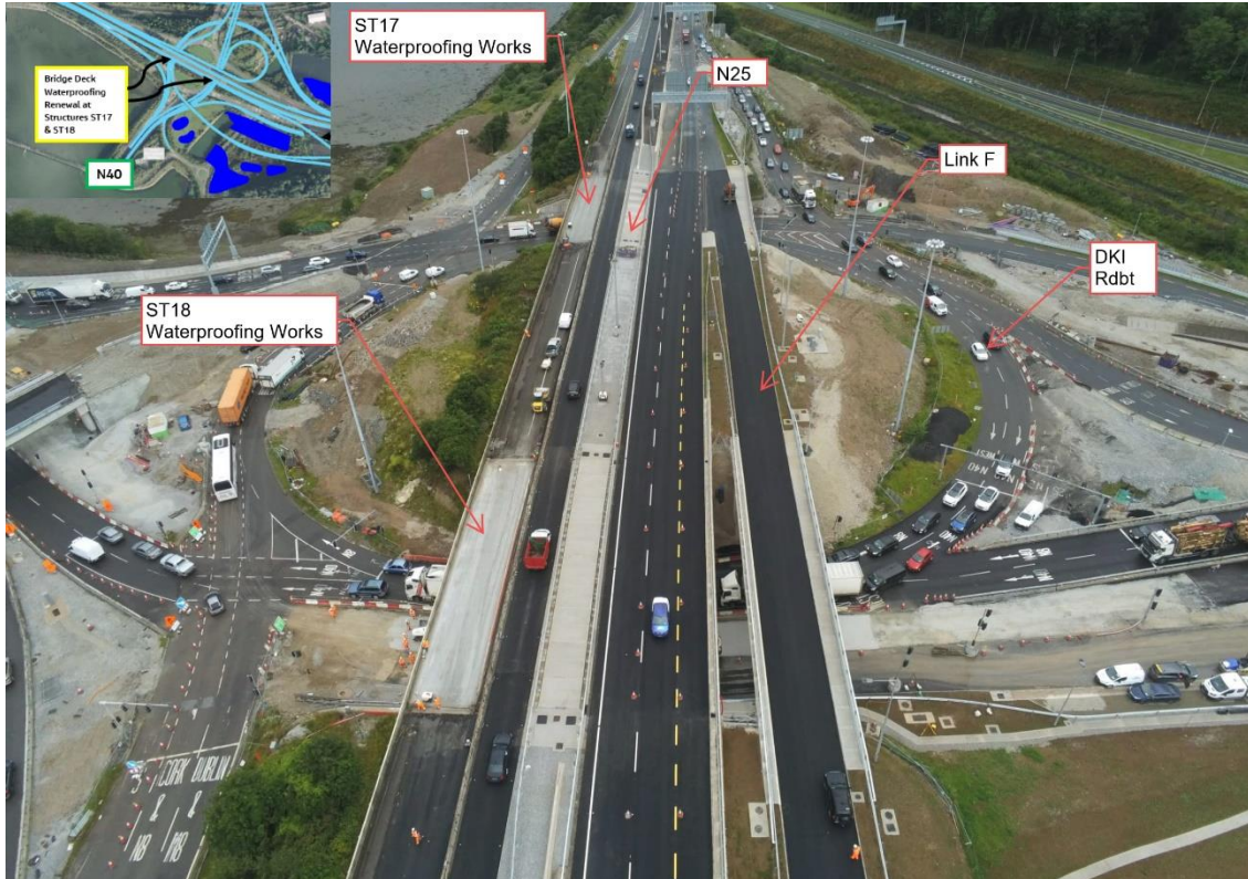
Preparatory works ongoing at the existing Interchange Structures ST17 & ST18 on the N25 westbound.
