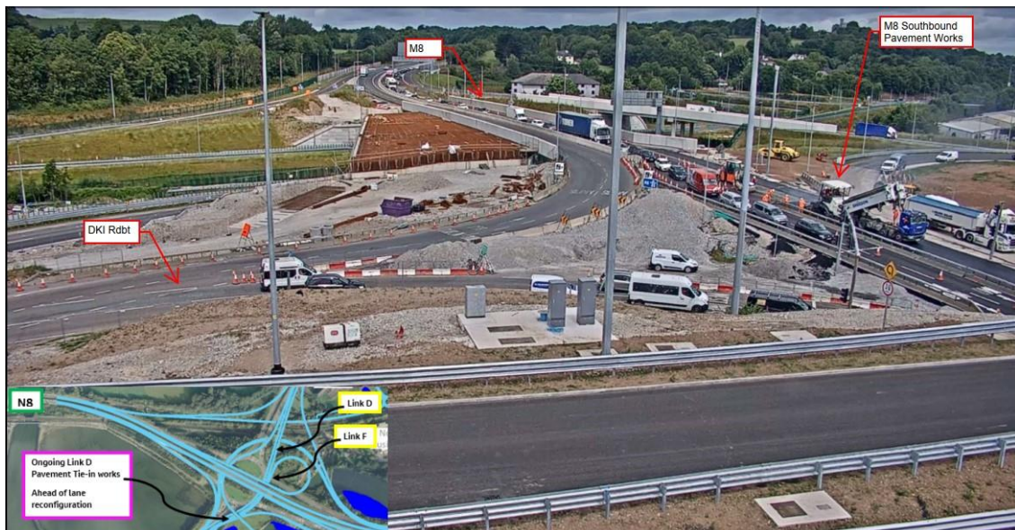
Surfacing works being progressed at the M8 Southbound approach to the DKI Rdbt.
