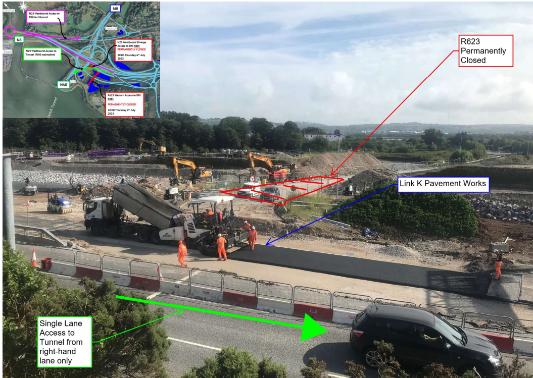
Pavement works ongoing at the intersection of Link K with the old R623 access to the Dunkettle Interchange Roundabout
