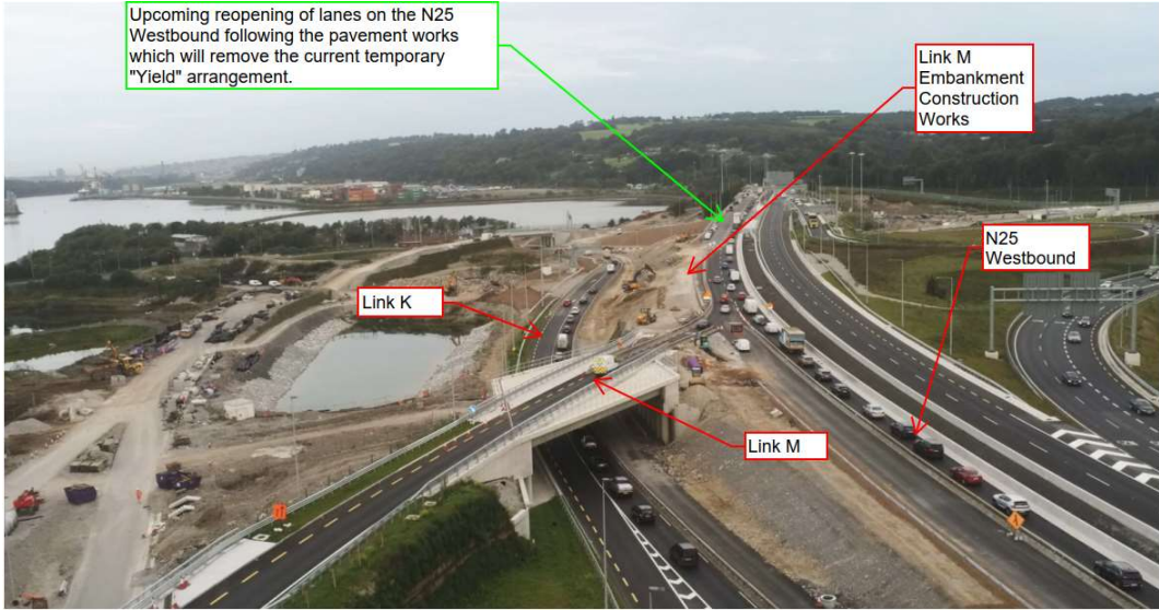
Ongoing construction of Link K and Link M alongside the N25 westbound
