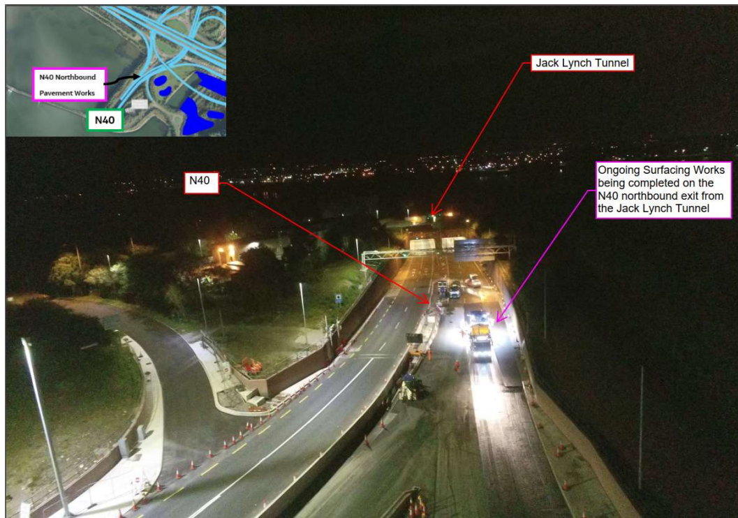
Pavement works ongoing on the N40 northbound directly north of the Jack Lynch Tunnel
